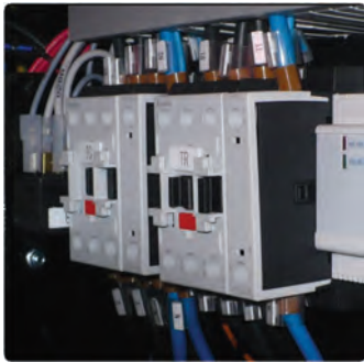
>> IN BUILT ATS PANEL
