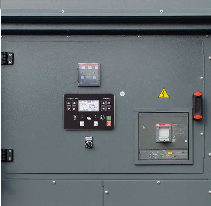
> Automatic panel with ComAp AMF8 control unit
