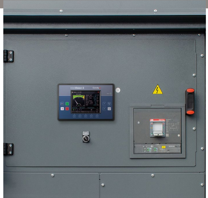
> Synchronization panel with ComAp IG1000 control unit
